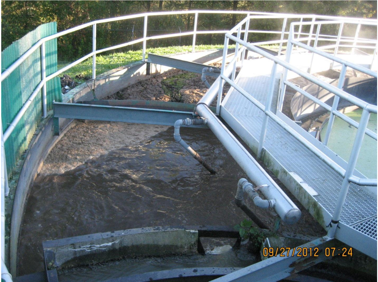
Photo: WWTP plant process component at Chalk River
