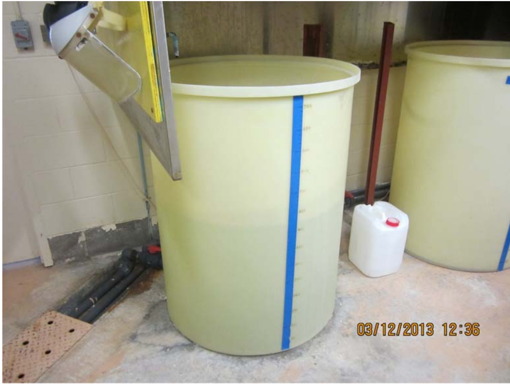
3) Chlorine storage vat
