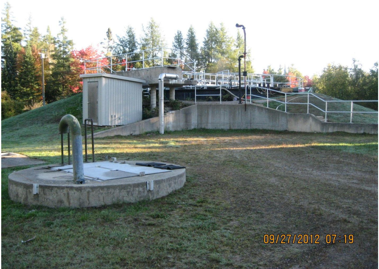
Photo: Chalk River Wastewater Treatment Plant above grade installation
